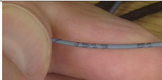
Figure 4 Cables are labelled with a fine print (rather than colour coded).
